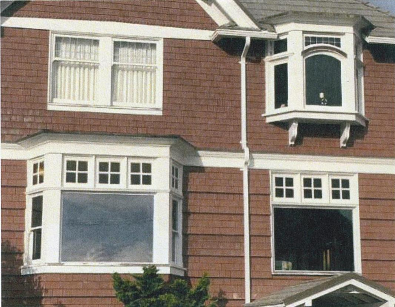
Weathered shingle siding, window frames need scraping, sanding and painting
