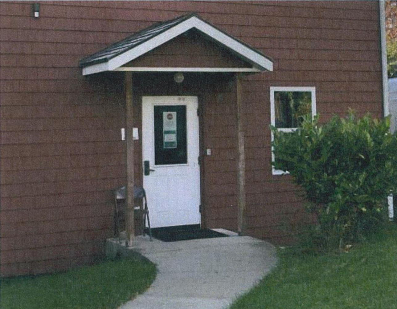
Landing outside of the Fellowship Hall entrance door does not have a code compliant clear floor area
