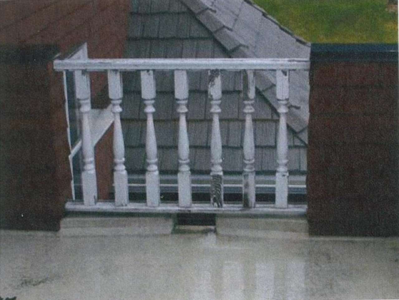
Balustrade on deck off Priest's office deck needs restoration and sealant under the door to stop water infiltration when the wind blows
