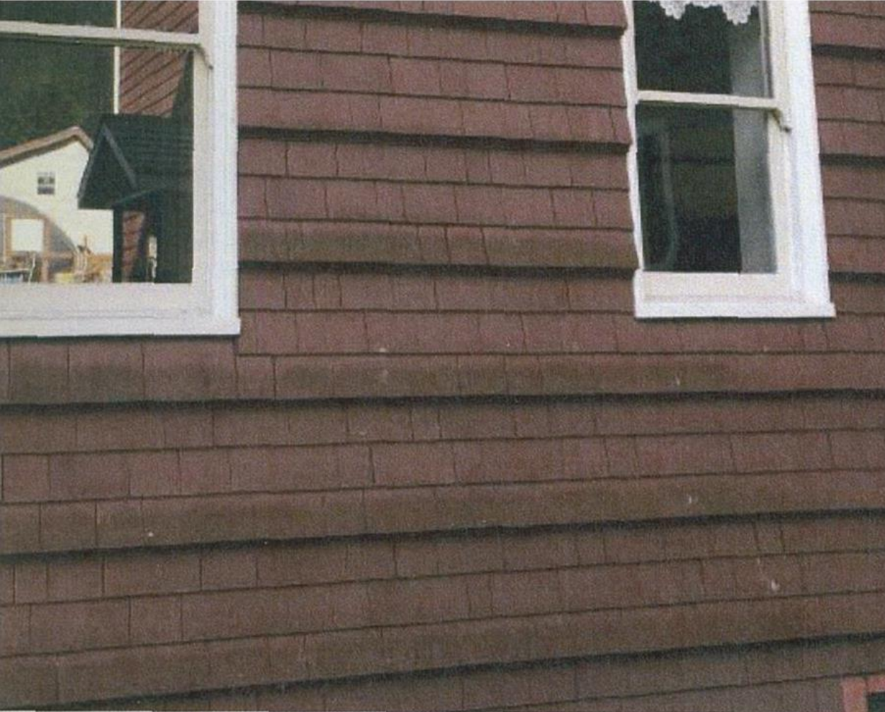
Mildew/soiling has accumulated on shingle siding, especially on the flared rows.
