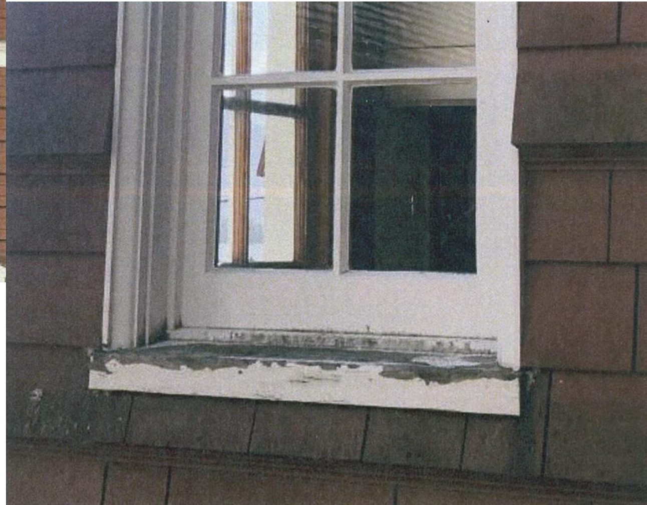
Window frame in Bishop's closet is in bad shape and rotted in some areas. Also need painting.
